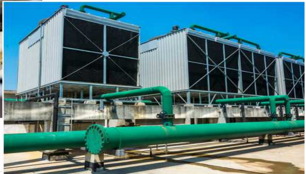
Air conditioning - commercial buildings
